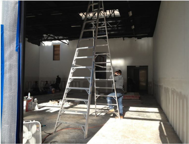
A week after Hurricane Sandy wrecked Chelsea's art district, 303 Gallery was fixing its flooded space. The damaged dry wall was removed. Photographer: Katya Kazakina/Bloomberg
